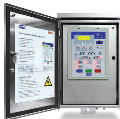
R200 protection relay cabinet
