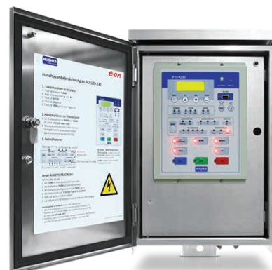
R200 protection relay cabinet
